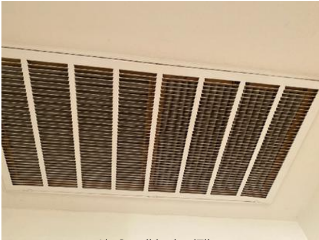
Air Conditioning/Filter Taken on: 2019-12-13 09:13:33 Image
