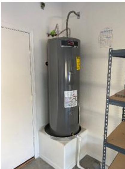
Water Heater Taken on: 2019-12-13 09:14:26 Image
